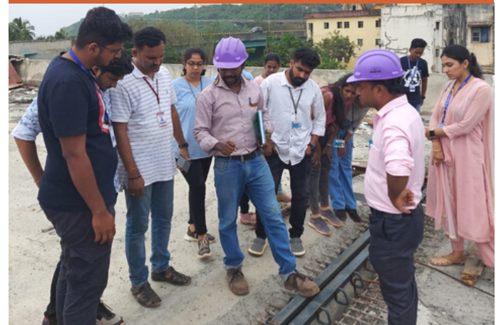
Field visit to Construction of Pylon nearby Baina Beach Vasco, Goa was arranged for M.Tech students on 4 th September 2023.
